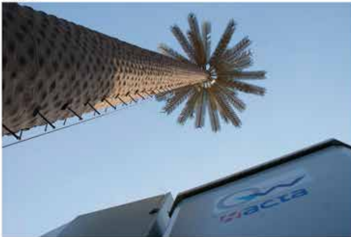
Acta Power installation in Cairo, Egypt
